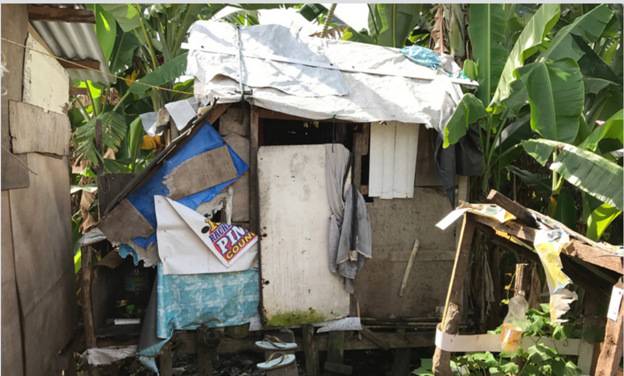
Clockwise from top: low-income housing rebuilt over the ocean in post-Yolanda Tacloban (2016); toilet facility through which human waste falls into the ocean, Tacloban (2016); a Tacloban home, three years after Yolanda (2016). Image credit: Rebekah Yore.
